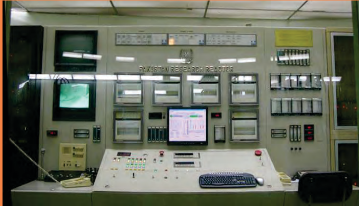
A view of PARR-I control Room
